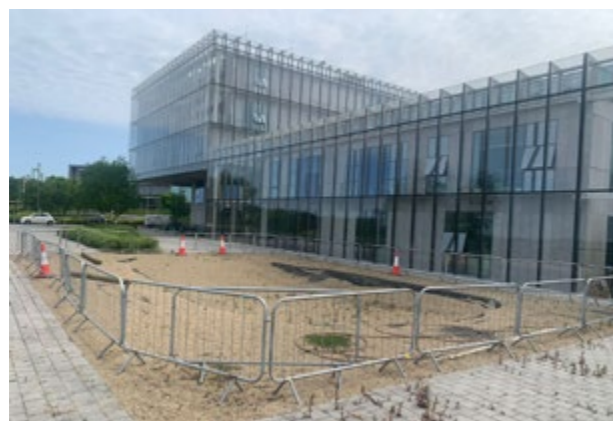
Figure 22: Collapsed Attenuation Tank - Wexford County Council
